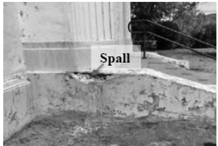
Example of the building's deterioration, Corri Jimenez Photo
